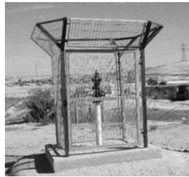
Fenced-off water pump at unrecognized village
